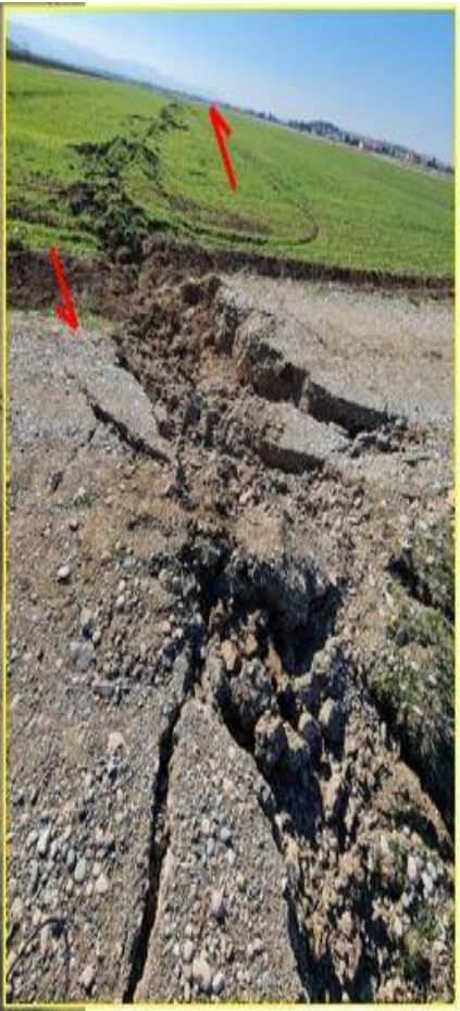
Two offsets on the road (photos 30 m apart) and fault surface rupture
